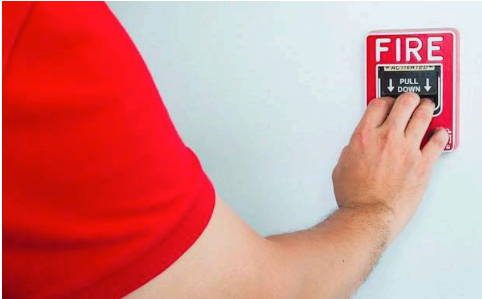
Gambar 6.2 Fire Alarm System atau sistem peringatan kebakaran. Sumber: CV Firechemindo Vincifire Protection/Vincifire.com/2022
