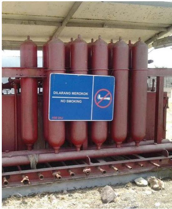
Gambar 6.28 Accumulator Sumber: Yudanto (2014)
