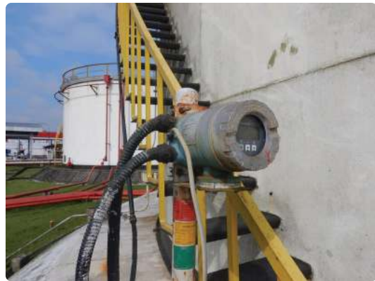
Gambar 8.9 Automatic Tank Gauging Sumber: Juwantoro (2023)
