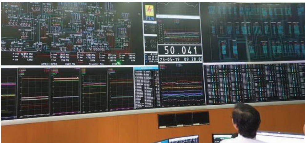
Gambar 1.14 SCADA Control Centre
